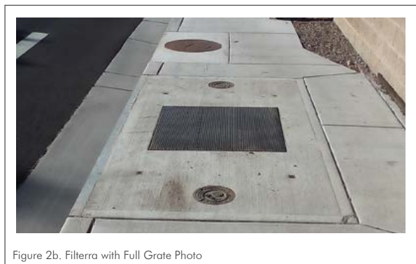
Figure 2b. Filterra with Full Grate Photo
